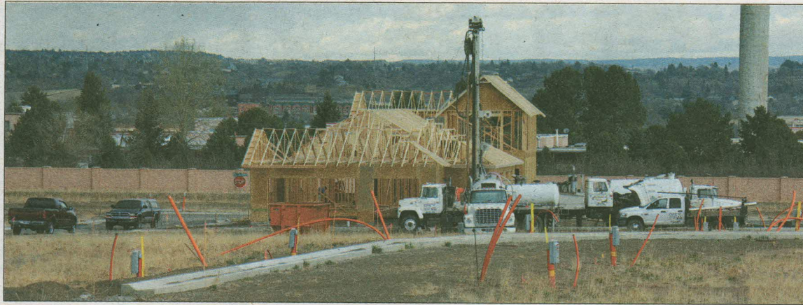
A drilling rig was creating three 340-foot holes this week to allow the geothermal service in the new G.J. Gardner model home being built at Gold Hill Mesa.
